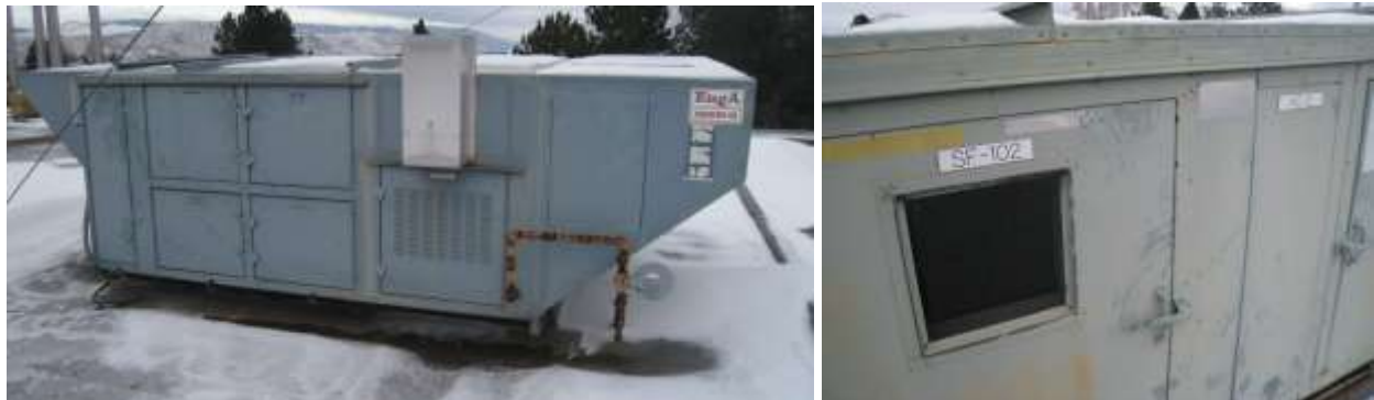
Figure 2.4: Makeup Air Unit & Air Handling Unit (SF-102)
