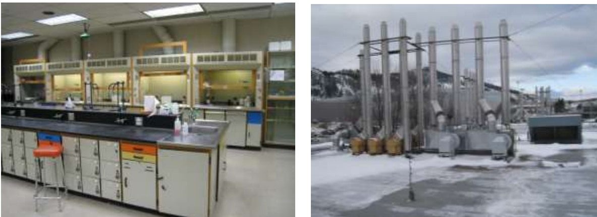
Figure 10: Fume hood exhaust and fans
