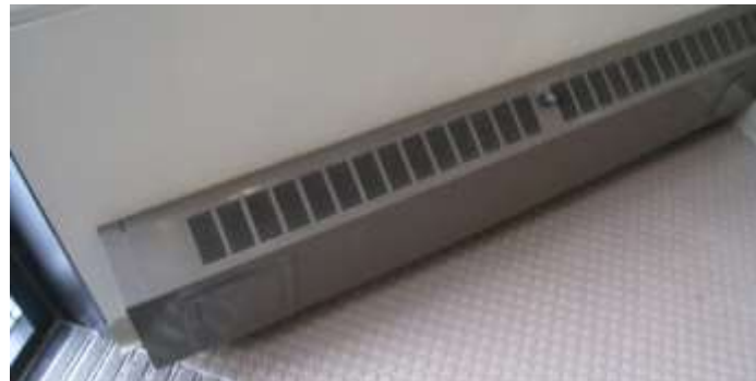
Figure 2.8: Wallfin Convectors in Stairwells
