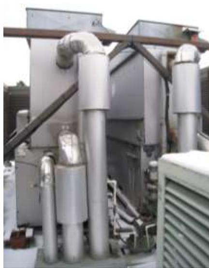
Figure 2.10: Fluid Cooler(s) located on roof
