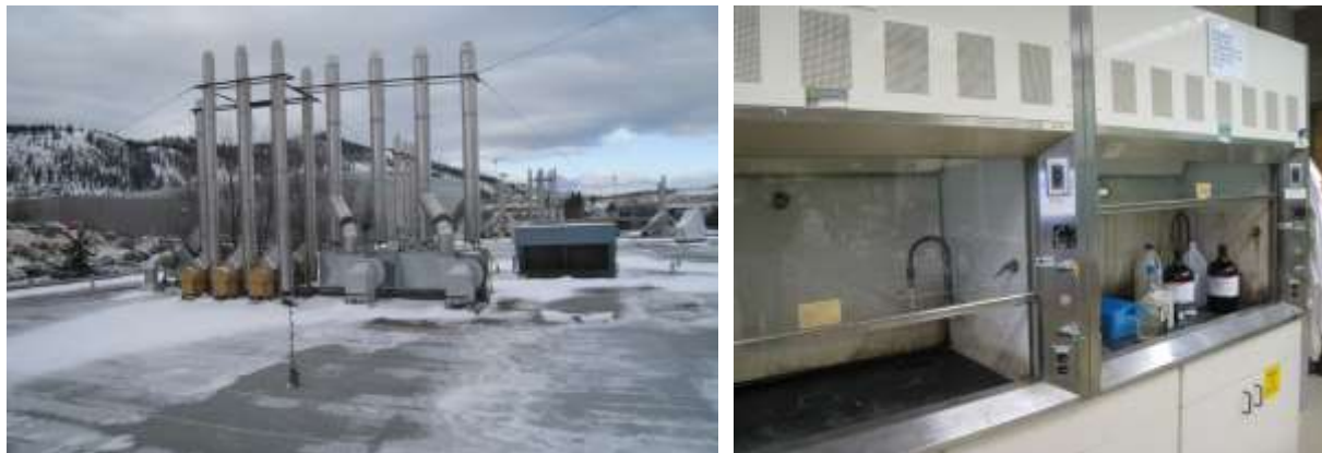
Figure 2.6: Lab Exhaust Fans and Fume Hoods
