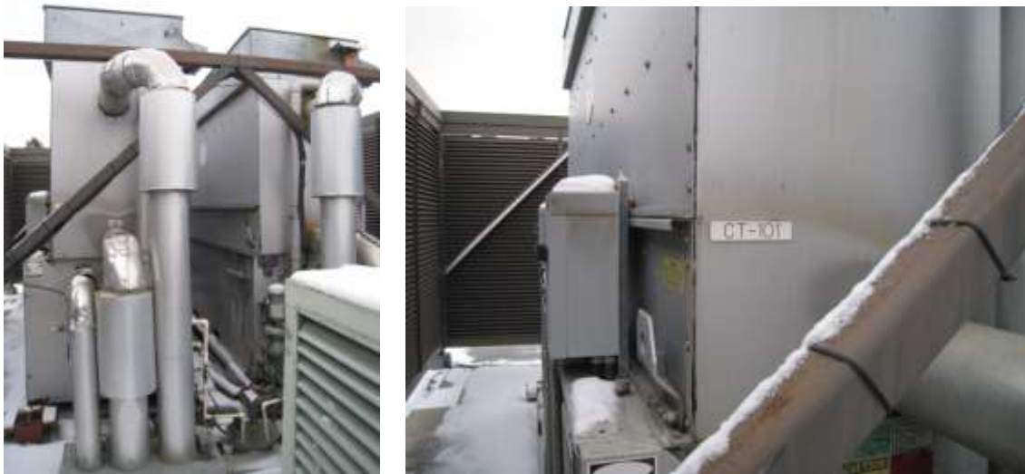
Figure 11: Cooling Towers located on the building roof
