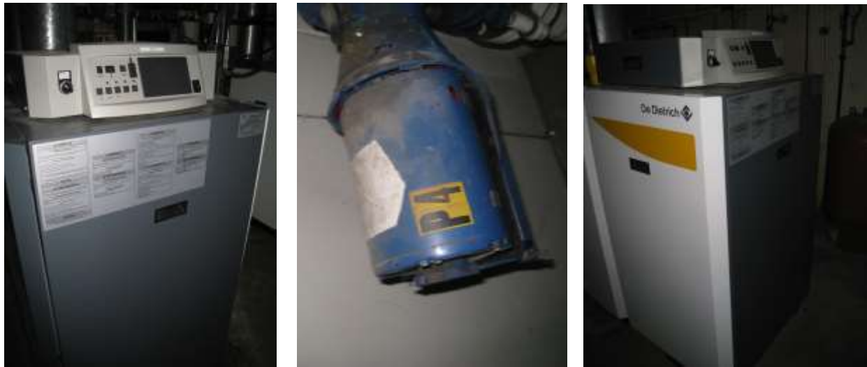
Figure 2.7: Existing De Dietrich Natural Gas Condensing Boilers & Circulation Pump P4
