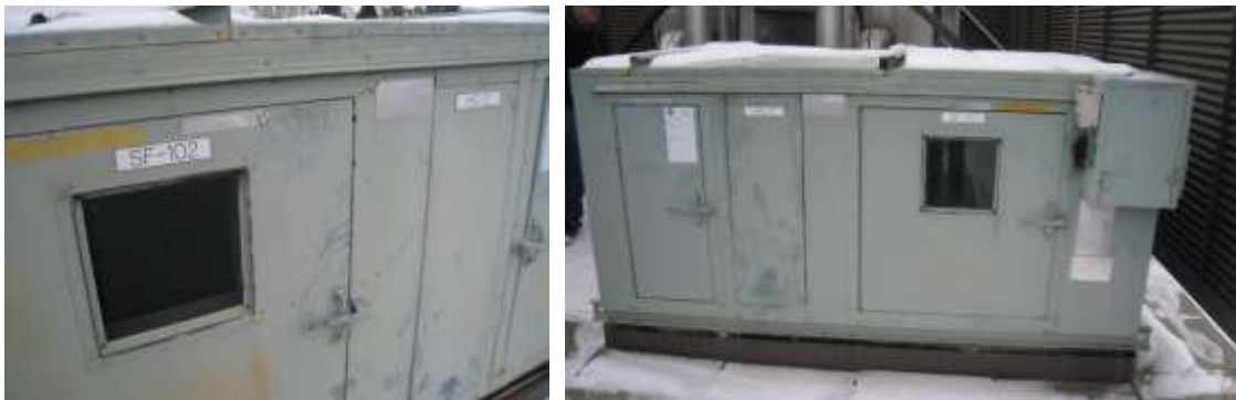
Figure 9: Air Handling Units SF-101 & SF-102
